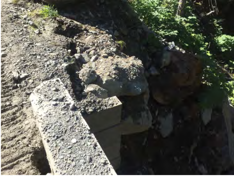
Downstream left bank fill erosion
