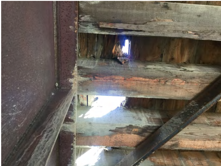
Hole in deck
