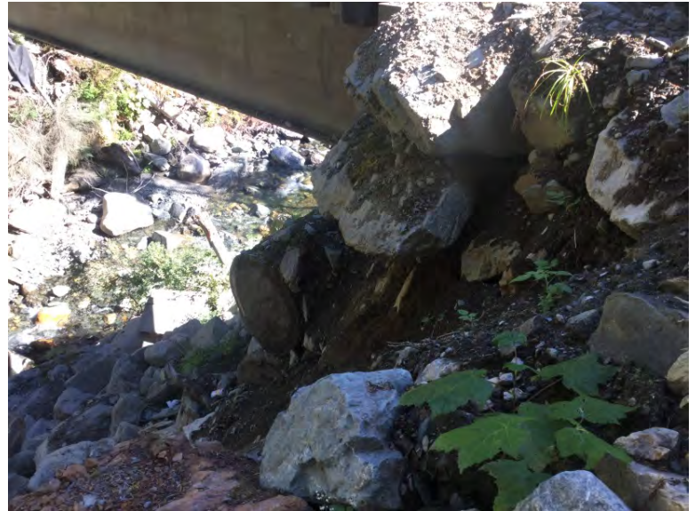
Downstream left bank fill erosion
